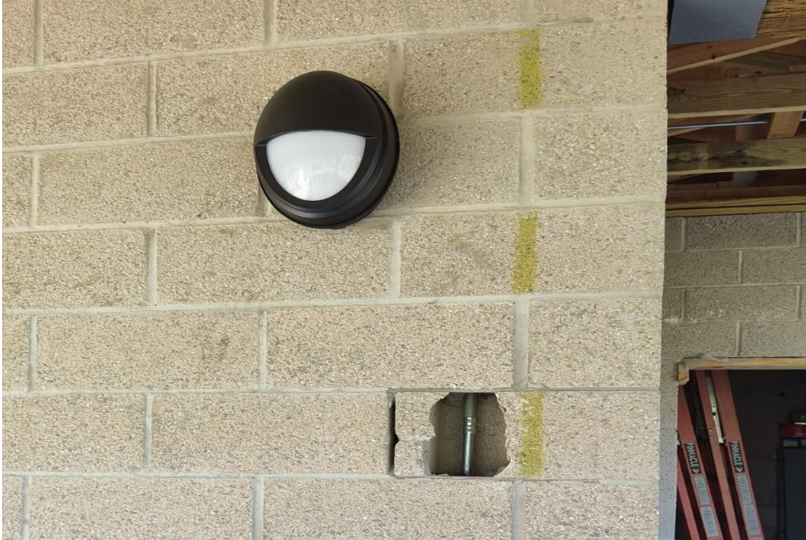
Photo 2: Exterior lighting installation, there was an issues with mortar in the conduit. As we can see the conduit has been replaced - block still unresolved and not replaced. Block still to be cleaned.
