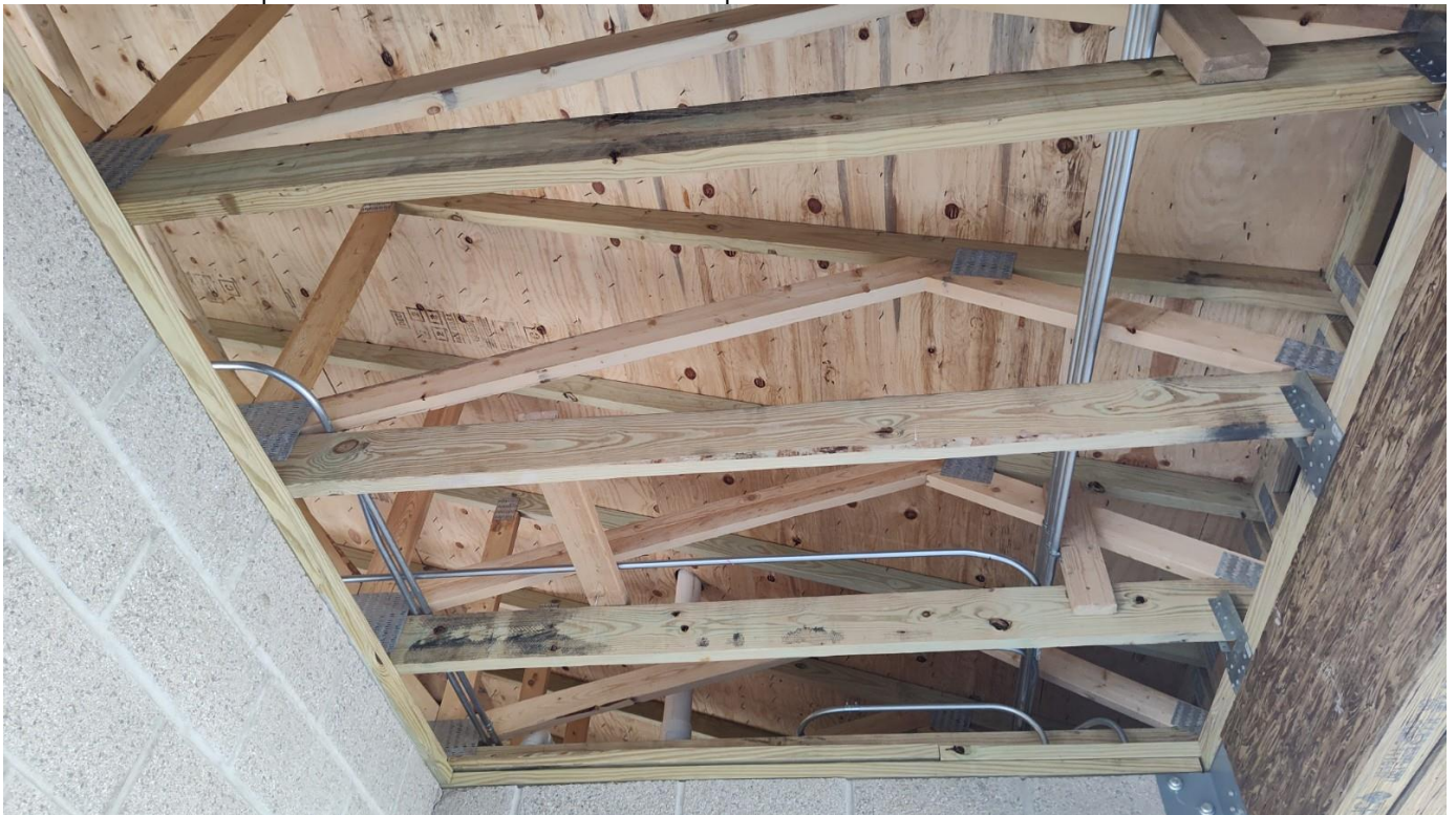
Photo 3: View of electrical conduit above.
