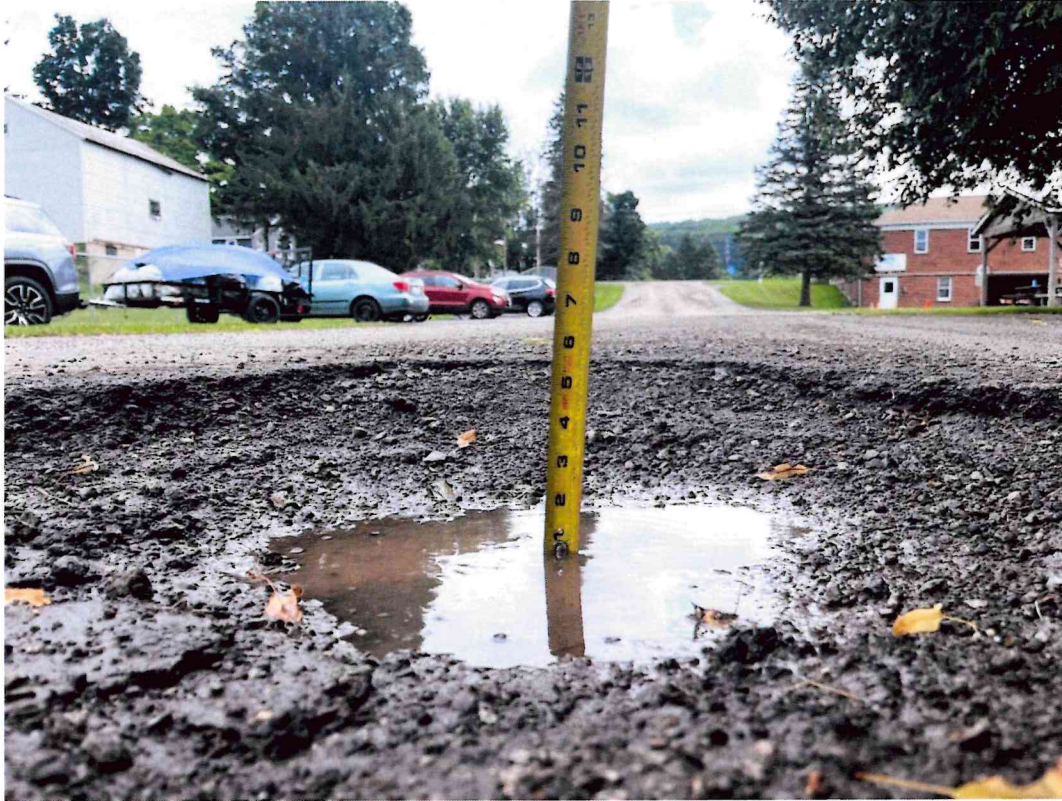
38" x 52" x 5.5" Deep Pothole:
