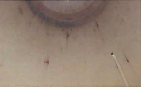
56. Corrosion on interior shell.
