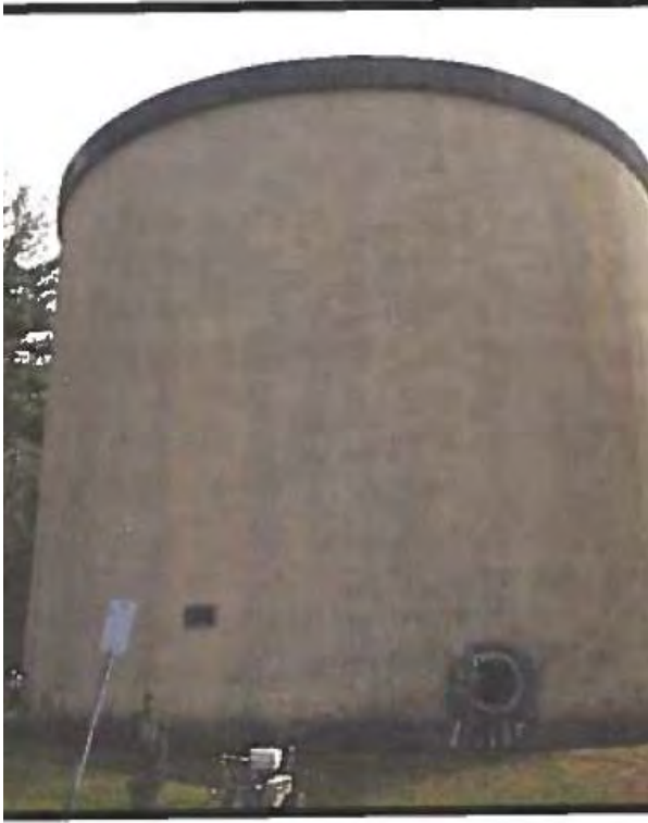
Water District 1 – Crestwood Tank
