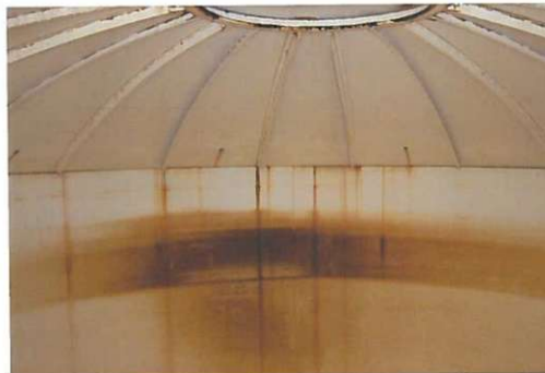
42. Roof and rust staining on upper shell.
