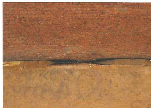
54. Voids in material along shell-to-floor connection.
