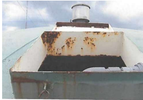
28. Corrosion on roof manhole.
