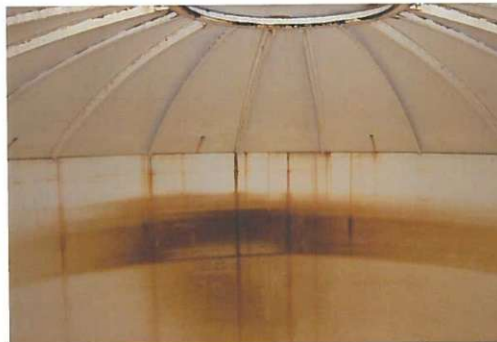
42. Roof and rust staining on upper shell.
