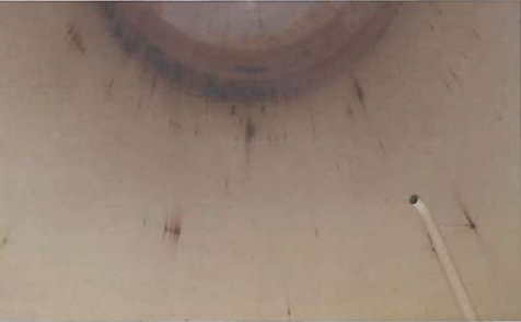
56. Corrosion on interior shell.
